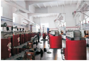
Test Bay for Dry-type Transformer
